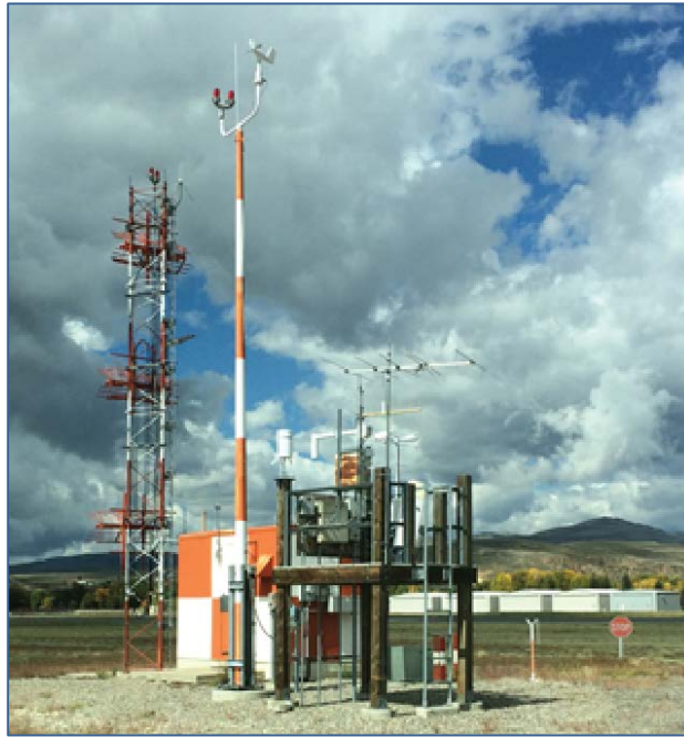
FIGURE 1-44 GLIDE SLOPE ANTENNA AND AWOS-3
